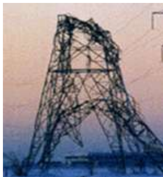
Figure 39-Devastated mighty Steel Structure after Montreal Ice Storm 1998 56
